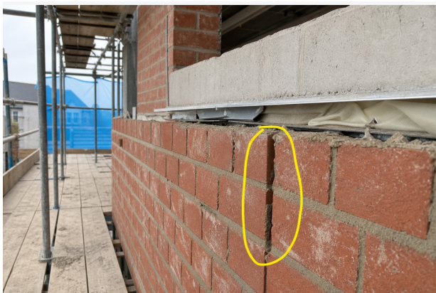
Open perp joint marked on the scaffold lift.
