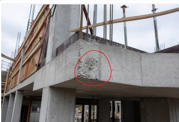
Honeycombing marked at the exposed concrete corner.
