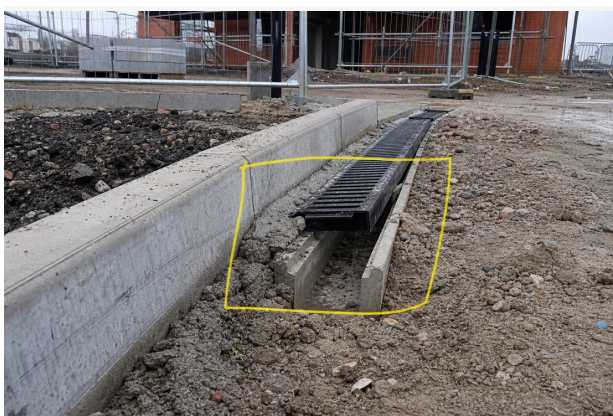
Loose channel drain cover and uneven haunching marked on site.
