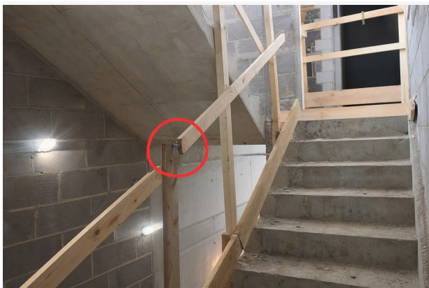
Temporary handrail fixing marked during stair core walk.
