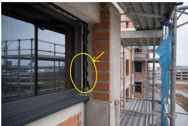
Window perimeter gap marked from the scaffold inspection.
