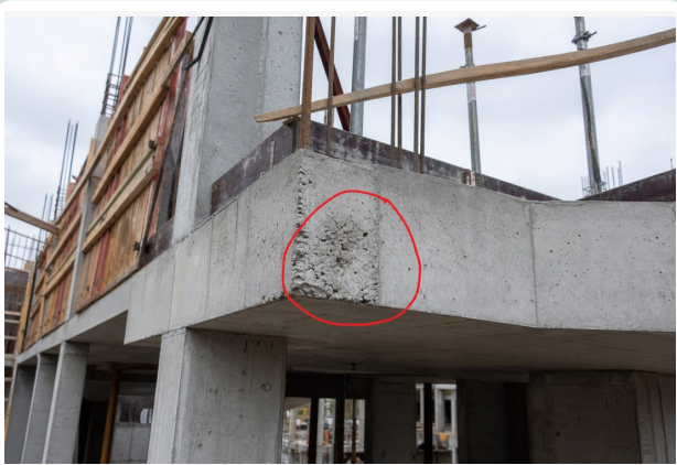
Honeycombing marked at the exposed concrete corner.
