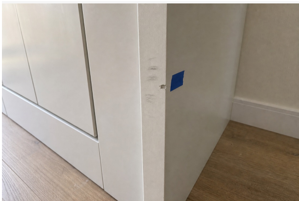
Paint scuff visible on the wardrobe return. Captured 2026-07-10 11:30 - SHA-256 6aa458e81f19bc3e (verified)
