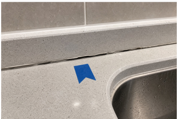
Gap visible behind sink upstand before sealant. Captured 2026-07-10 12:30 - SHA-256 159279d98a7adfa2 (verified)
