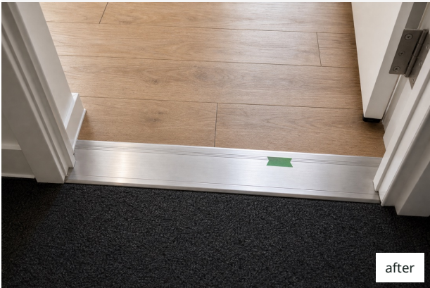
Threshold polished and accepted at reinspection. Captured 2026-07-10 10:30 - SHA-256 e4ca61ec141f342b (verified)
